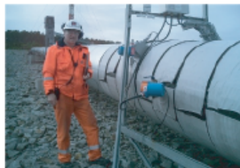
▲ On pipe 42" flare gas
