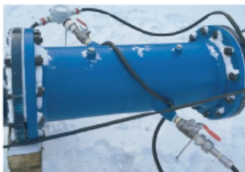
▲ 12", flare gas, drilling rig
